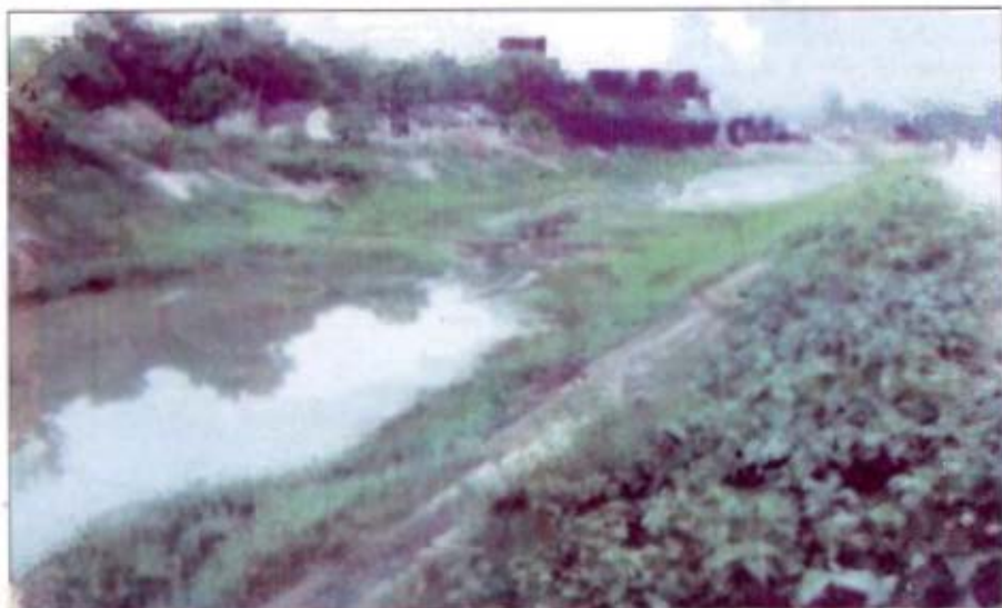
Siltation and vegetation in WKMC at RD 135.45 Km (BIHAR)
