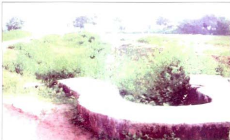
No water and need for bush clearing at Chainage 319 km of Tapkara Project (JHARKHAND)
