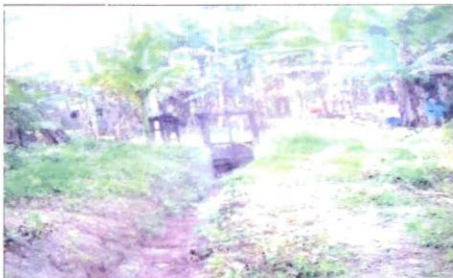
Gandual MI Project—Cross Regulator in the earthen canal with no water (MEGHALAYA)
