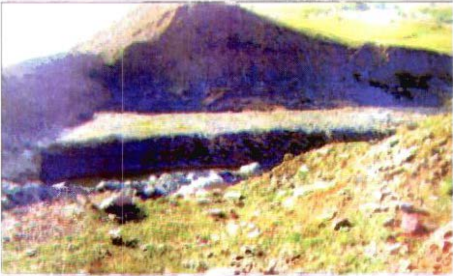
Incomplete spillway of Nayaki Reservoir Scheme (BIHAR)
