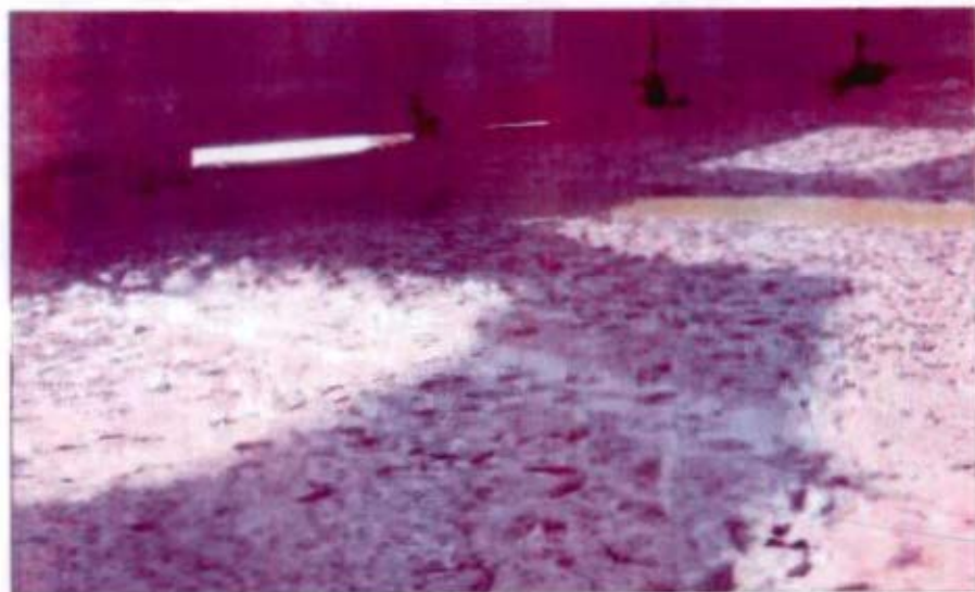
Siltation in upstream of Western Kosi Main Canal (WKMC) at RD 55 Km (BIHAR)
