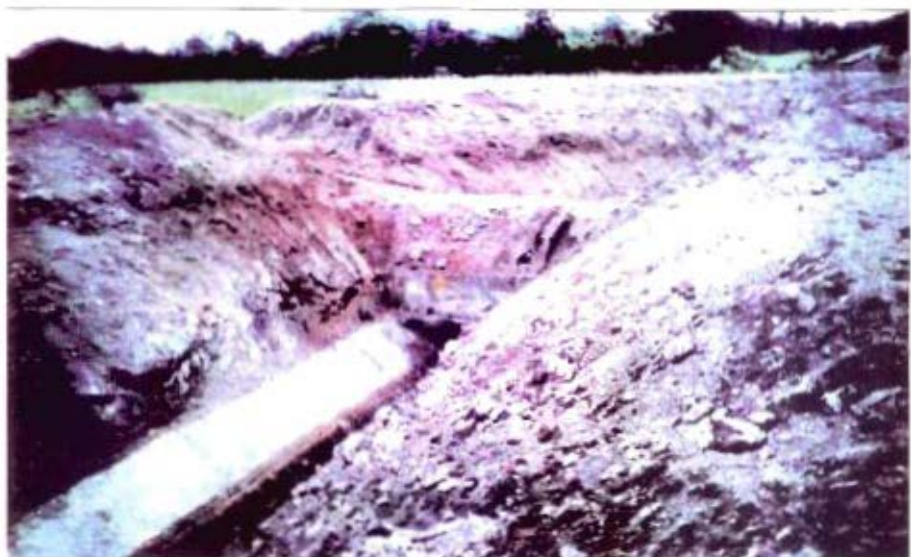
Bottleneck in tail end of Almutti Left Bank Canal of Upper Krishna Project Stage II (KARNATAKA)
