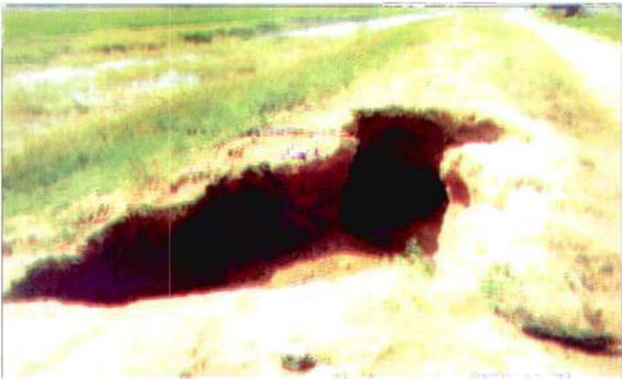
Damaged embankment of Gerua Reservoir Scheme (BIHAR)
