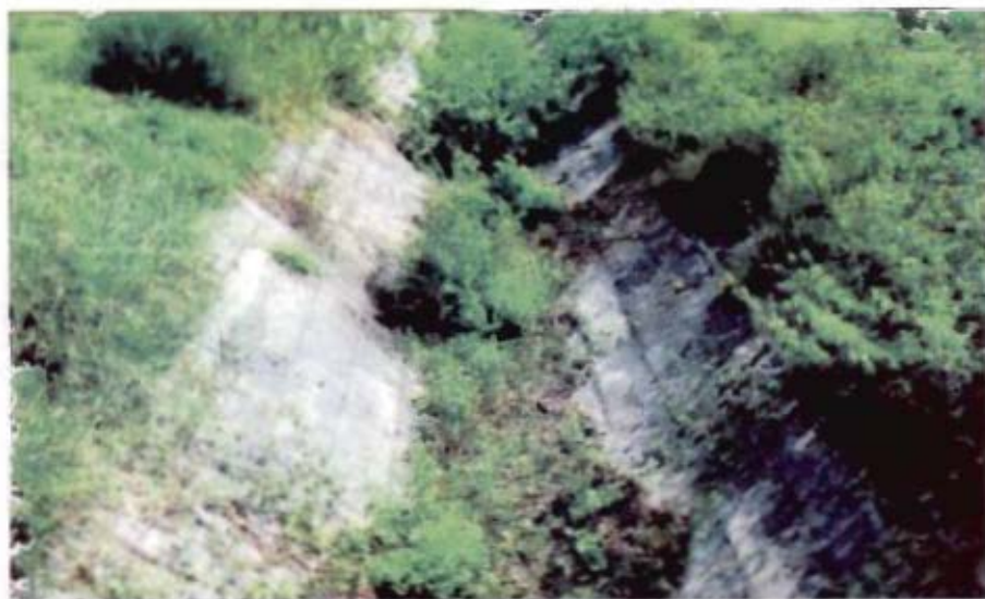
Mukteshwar Project-Dry canal with Weeds and Siltation (GUJARAT)
