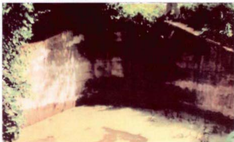
Thoubal Multipurpose Project—Non-functional canal syphon at RD 25.518 km. (MANIPUR)
