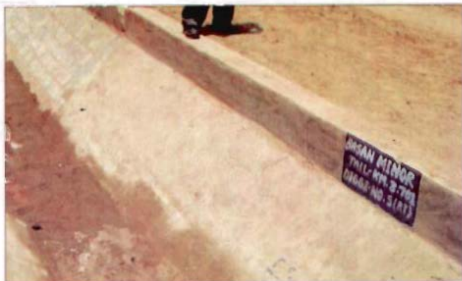
Narmada Canal Project – Incomplete work in the Inlet of Diggi No. 5 Basan Minor at tail 3.701 km – Vank Distributory (RAJASTHAN)
