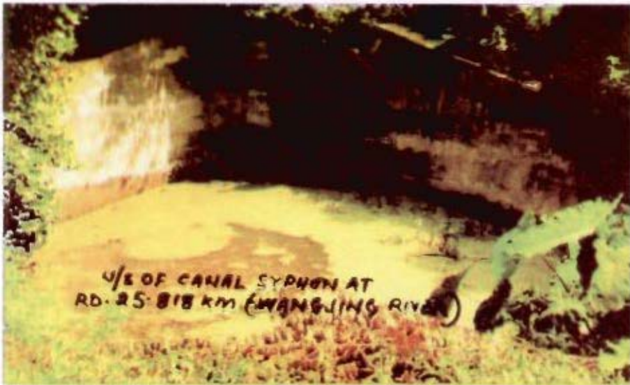
Thoubal Multipurpose Project – Manipur: Non-functional Canal Siphon (MANIPUR)
