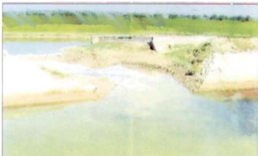
Western Kosi- Bihar - Breakage in Saharghat Branch Canal (BIHAR)
