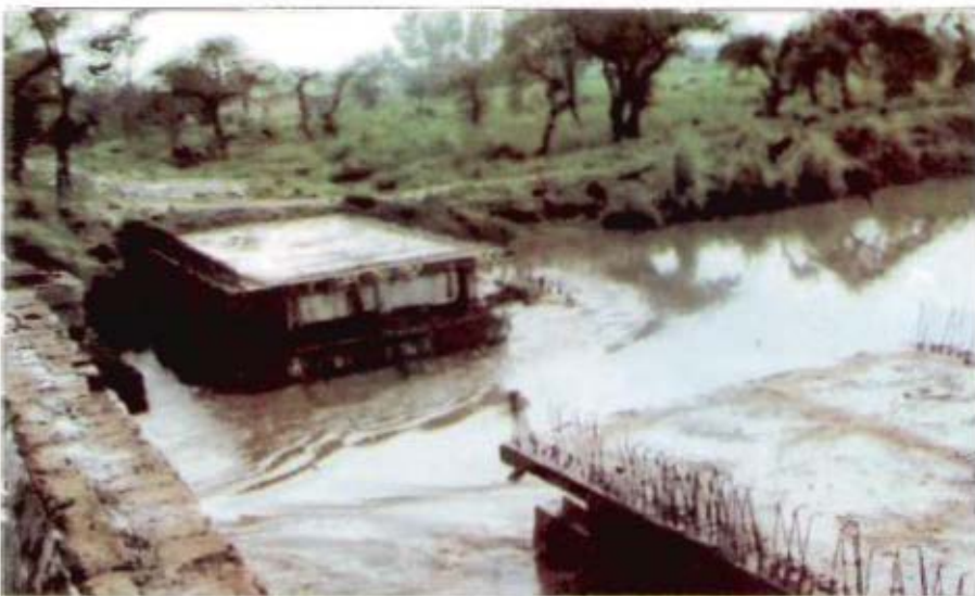
Agra Canal Project – Uttar Pradesh: incomplete bridge at Chhajunagar (despite the fact that the project was declared as completed) (UTTAR PRADESH)
