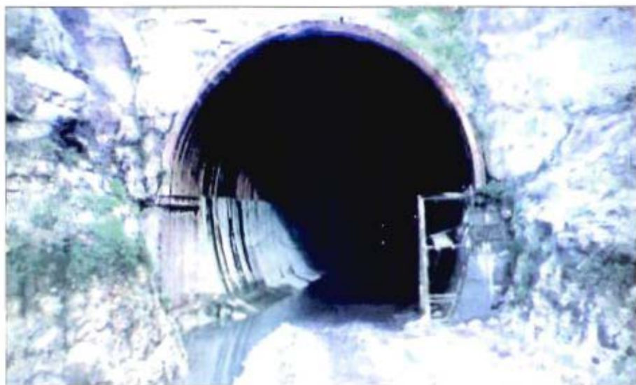
Incomplete tunnel work at road 33 to 35 km of Bargi Diversion Project - Ph-I (MADHYA PRADESH)
