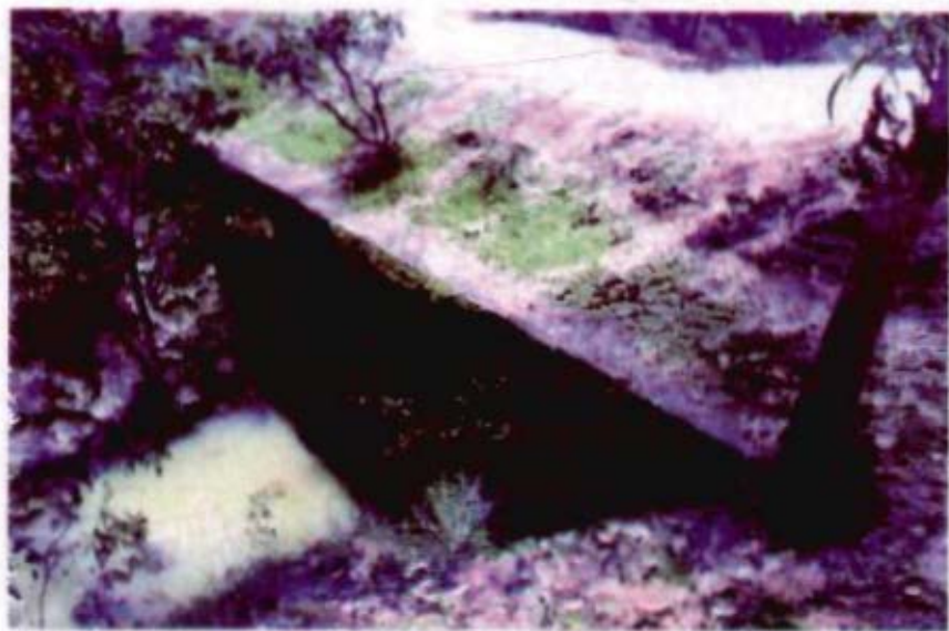
Chainage 199.89m beyond which actual bed level was higher than the design bed level in Purulia District. Resultantly there was no flow of water. (The water in picture is rain water) (WEST BENGAL)
