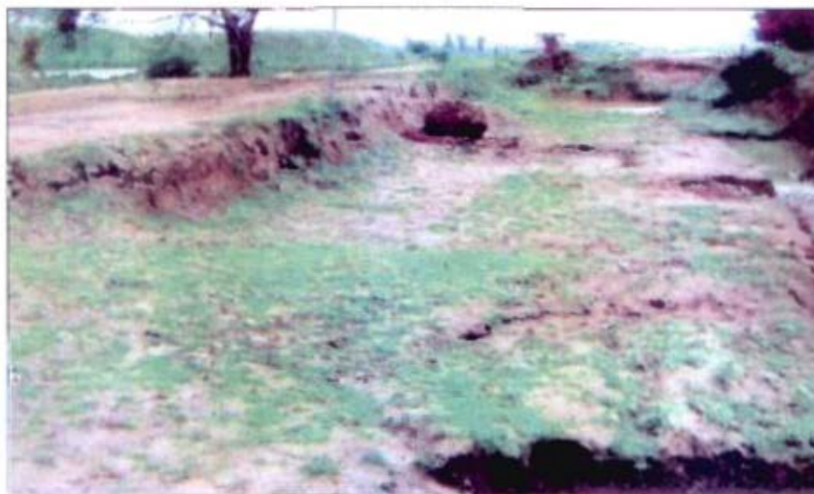
Sone Canal Modernisation Project (SCMP) – Bihar : Incomplete Western Parallel Link Canal (BIHAR)
