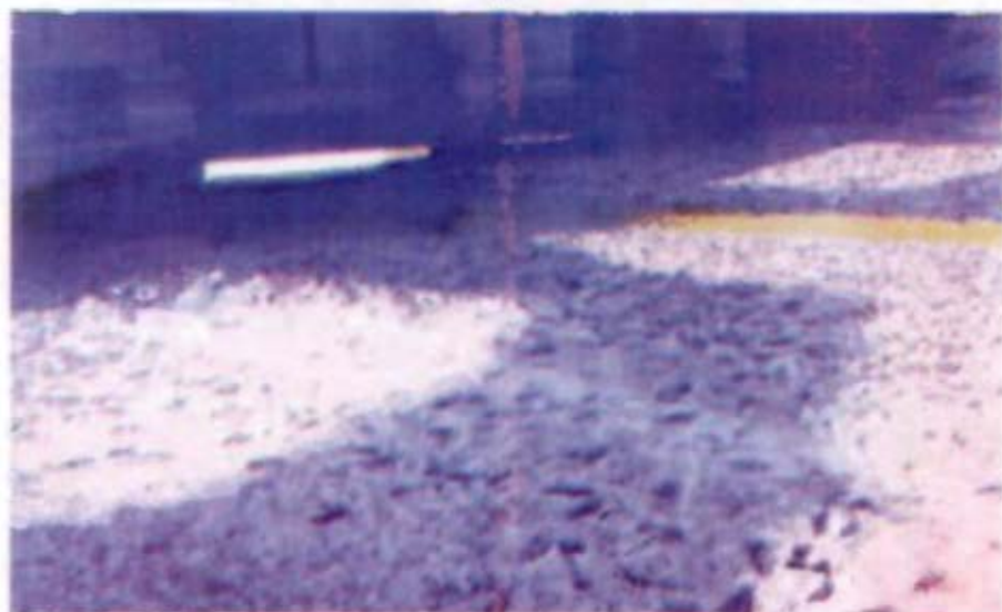
Western Kosi Main Canal - Bihar : Siltation in upstream (BIHAR)
