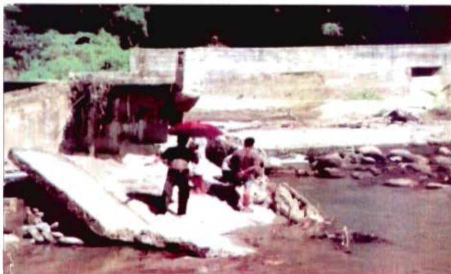
Damaged headwork at MI Projection Kanabung Village, Itanagar Division (ARUNACHAL PRADESH)
