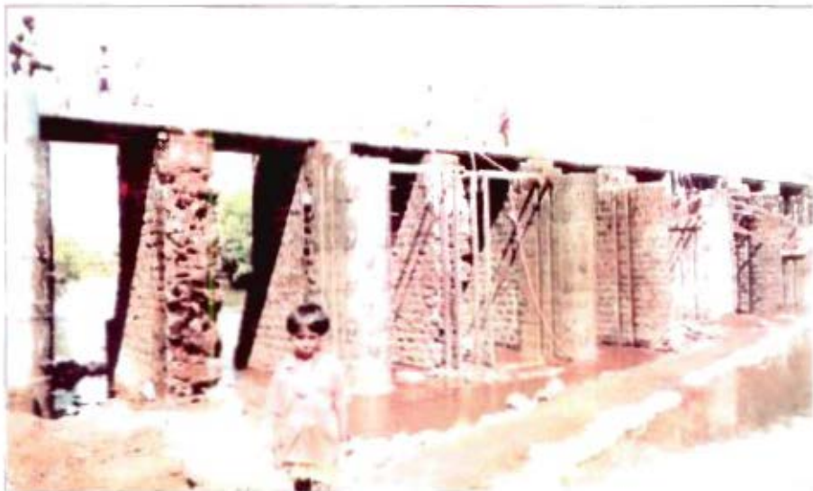
Repairs to the existing KT weirs in Patgaon Medium Project yet to be carried out (MAHARASHTRA)
