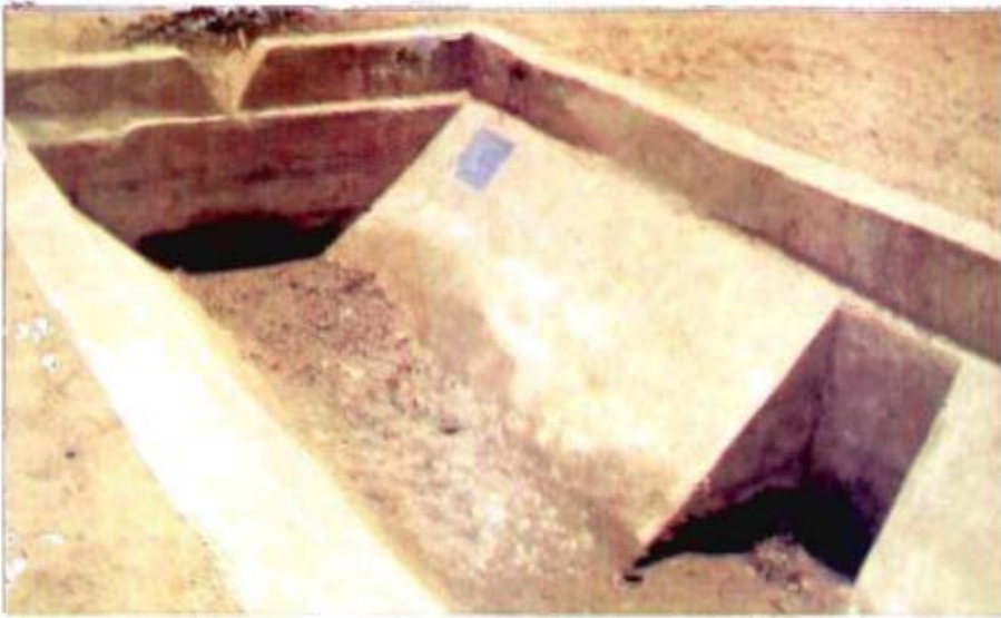
Narmada Canal Project – Incomplete work in the Inlet of Diggi No. 5 Basan Minor at tail 3.701 km – Vank Distributory (RAJASTHAN)
