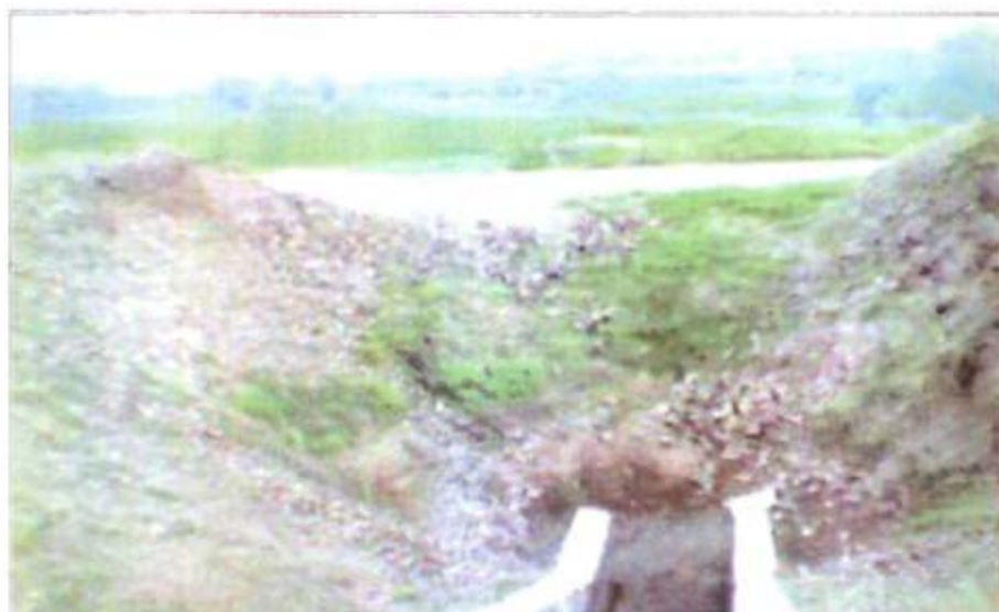
Bansar Project (Unit II Canal) – Madhya Pradesh : Sihawal Canal - Incomplete Structure at Rd. km. 42 (MADHYA PRADESH)
